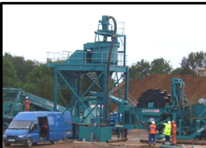
Lignite Removal Plant
